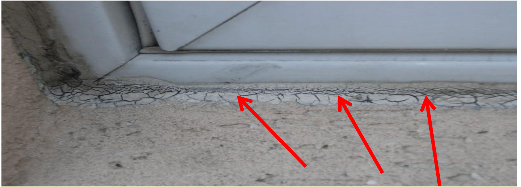
Cracked PU(Polyurethane) Sealant (Window Perimeter Joint)
